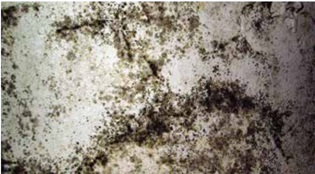
Mould growth is a common problem in damp and moist environments
